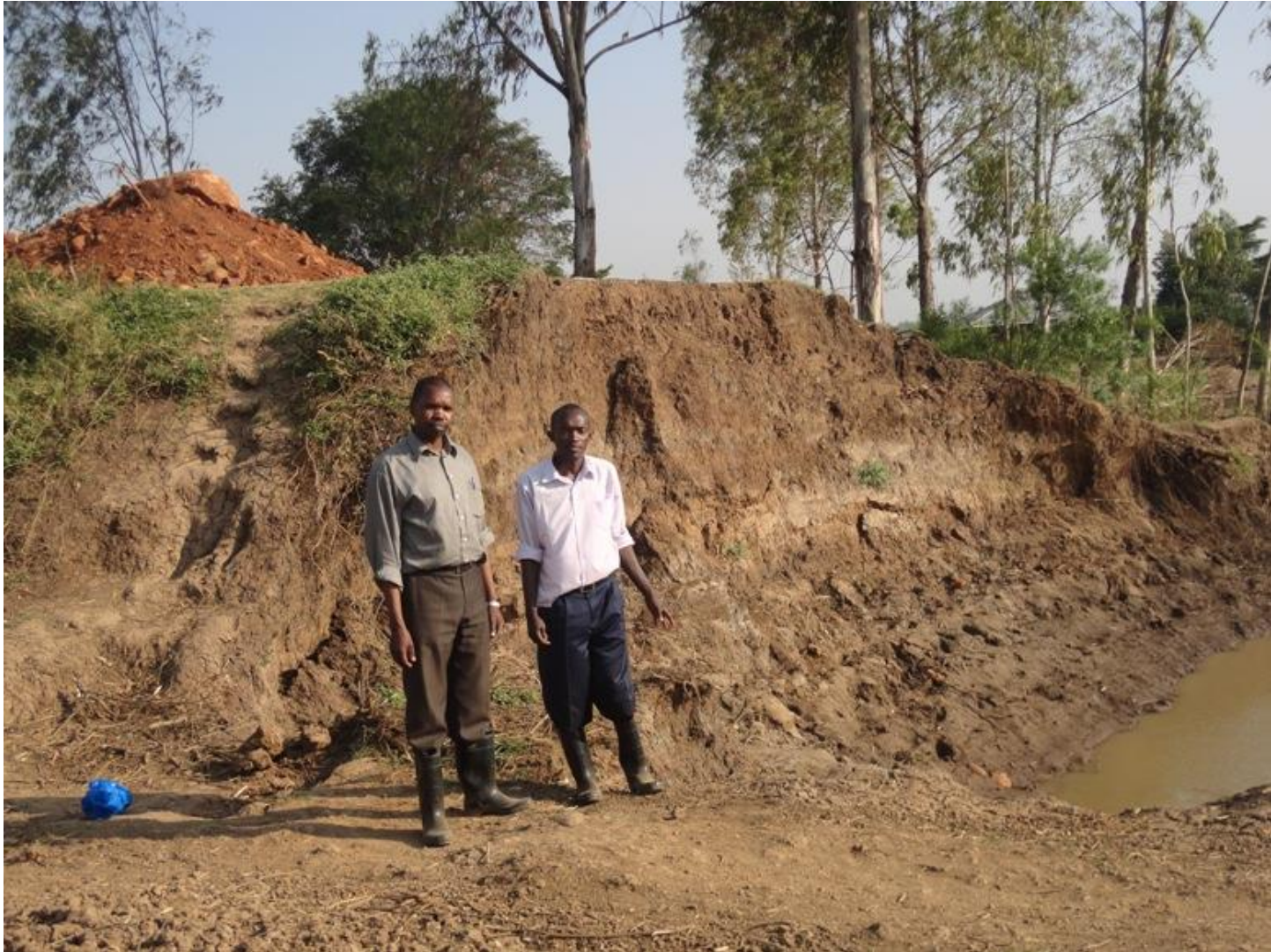
During a Survey to a breached dyke in Jan 2012
