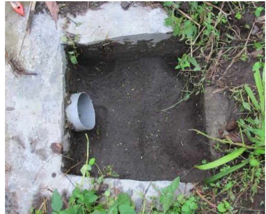
Infiltration pond at pine forest area. Control box, about 40% , was filled by sediment
