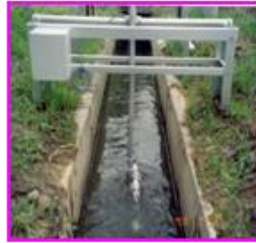
Flow meter & logger
