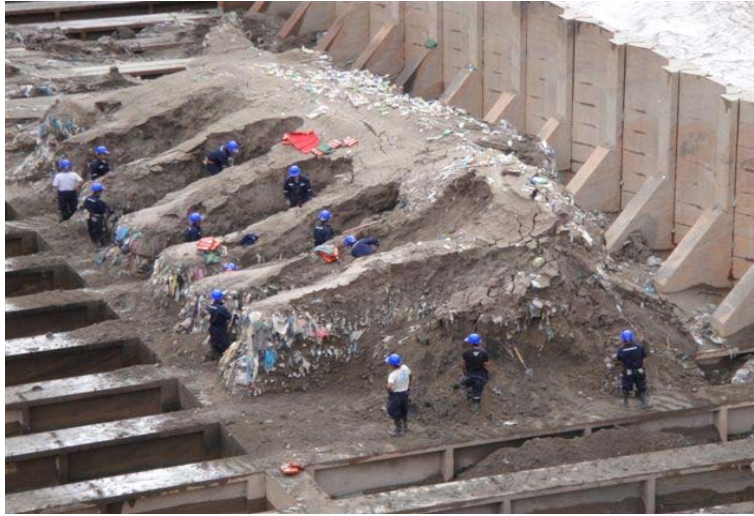
Fig.1 Sedimentation and desander cleaning works in the reservoir of Tablachaca dam situated some hundred kilometers upstream of Cerro del Águila dam From (Arbolí Nevot et al, 2018)
